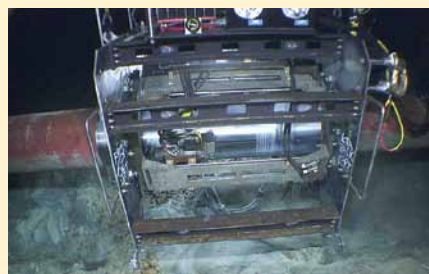
The weld seam and Fusion Bond Epoxy (FBE) removal tool used subsea to prepare the HOOPS pipeline for adding a tie-in connection. Photo courtesy of Shell
