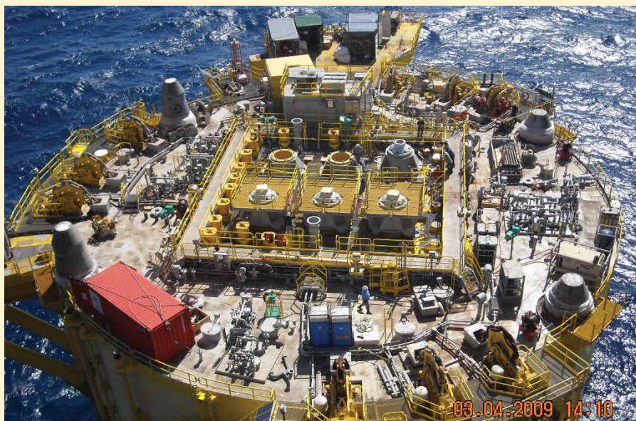
Perdido spar riser tensioners in various stages of installation prior to installation of the topsides. The six tensioners are in two rows in the center square of the spar deck. The three units on the bottom row are installed complete and stroked down (closed) awaiting commissioning. The remaining units on the top row are in various stages of installation.
