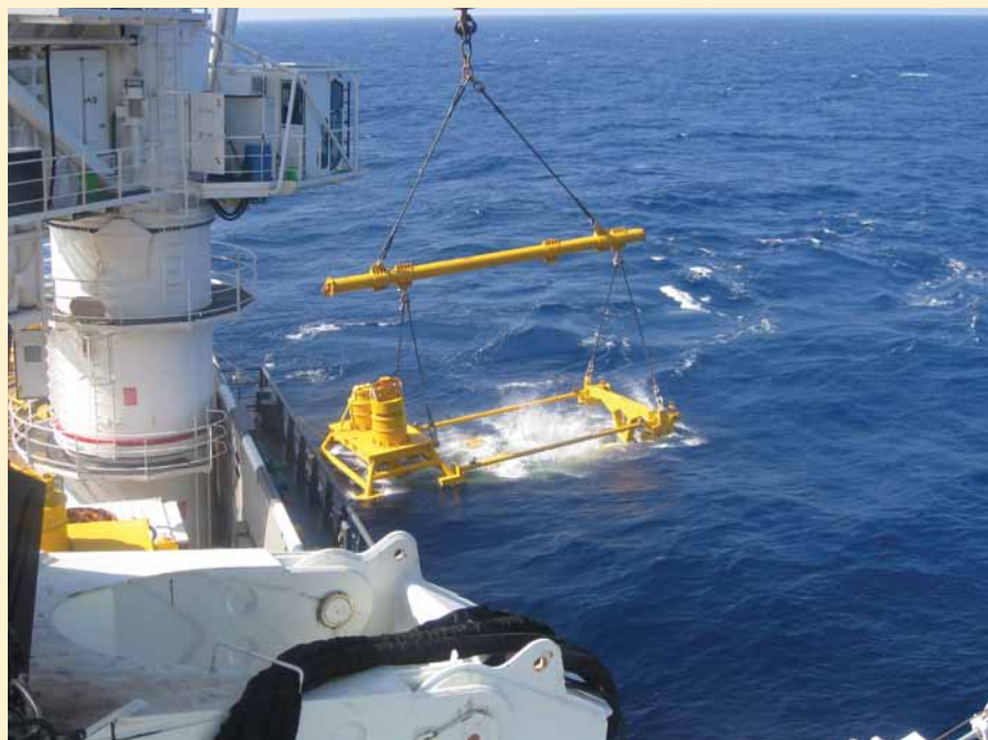
Oceaneering lifting the dual-hub connection assembly using the 150-mt active heave-compensated crane on the deck of the Olympic Intervention IV .
