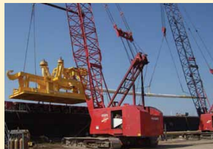
Perdido PLET sled S-2 and a double-jointed flowline with FBE and GSPU coating loaded to barge.
