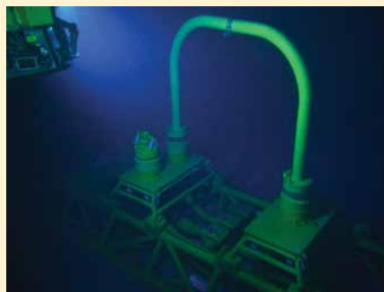
Millennium® Plus ROV surveys the completed jumper installation and subsea tie-in at 4500 fsw.
