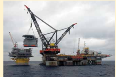
Heerema Marine Constructors' semisubmersible crane vessel (SSCV) Thialf engaged in making Perdido spar's Quarters lift.
